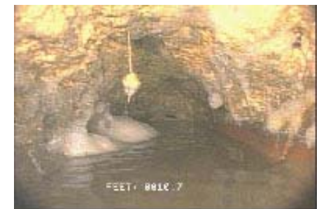
Grease on walls of a sewer pipe
